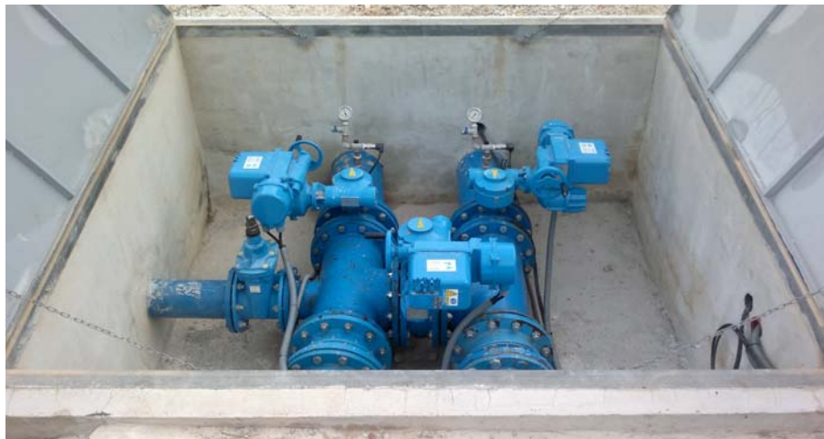
Figure 7. Valves are utilized to control, regulate and protect the network.
