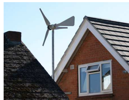
Picture. Domestic wind turbine [Ref. 40]
