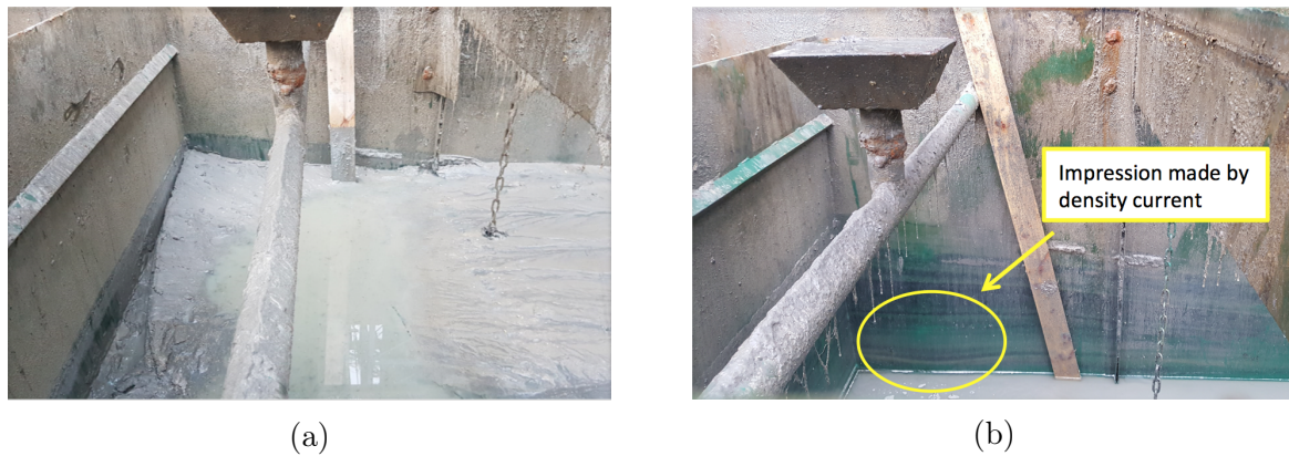
Figure 2.9: Interior photo of MEL5 between Stage 1 wall and Baffle 1 (a) Before desludging (b) After desludging with visible stratification marks on wall
