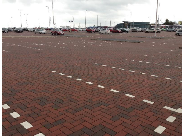
Figure 2. Permeable pavement implemented in Dunfermline, Scotland. (Photo taken by Ignacio Andrés Doménech).
