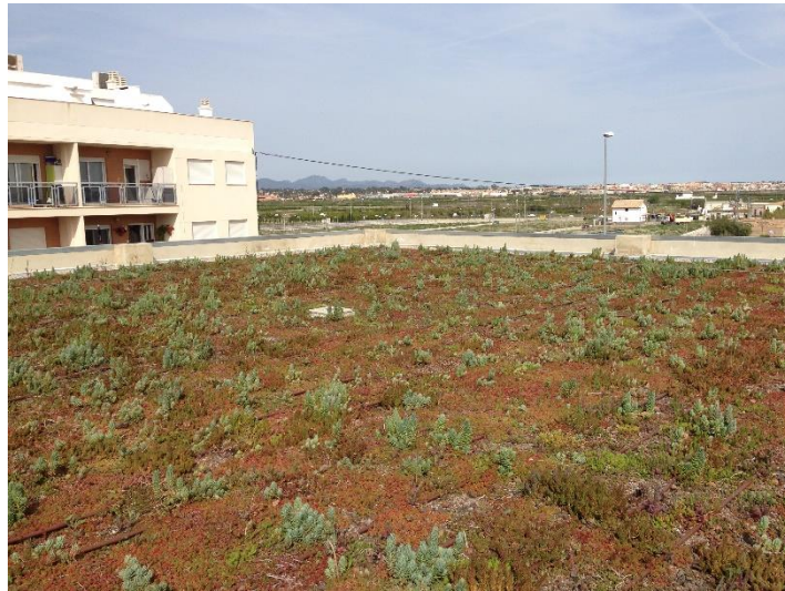
Figure 1. Green roof implemented in Benaguasil, Spain. (Photo taken by Ignacio Andrés Doménech).
