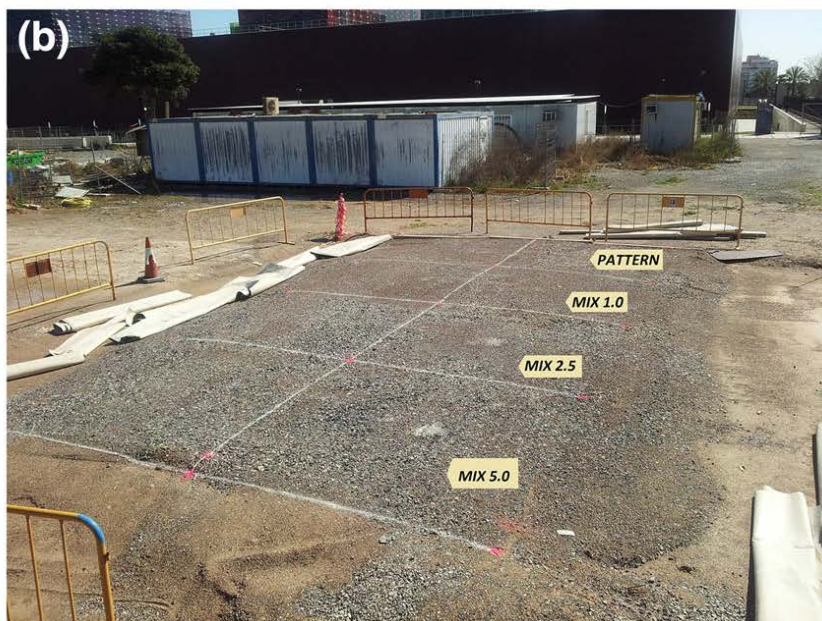
Fig. 2: Experimental railway platform. a) Platform layout (the vertical dotted line represents the track central axis). b) Completed platform
