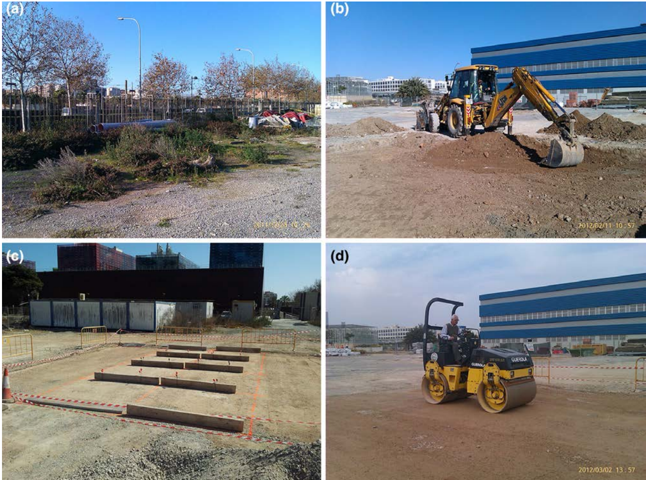
Fig. 3: Experimental platform construction process. a) Site before cleaning and clearing. b) Excavation. c) Site survey. d) Placing and compaction
