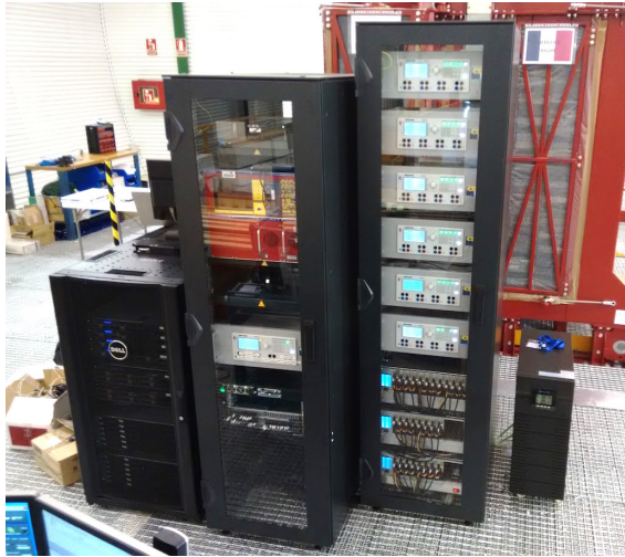
Figure 1.24: The NEW electronics cabinets. From the left, the computers and servers, the energy plane, and the tracking plane cabinet. At each side of the cabinets there is a big UPS, capable of supply the whole system up to 40 minutes in case of power failure.
