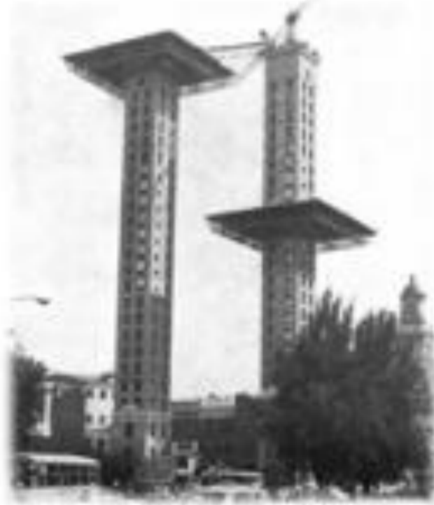
5. Lifting of the formwork by bars and climbing jacks in "Torres de Colón"
