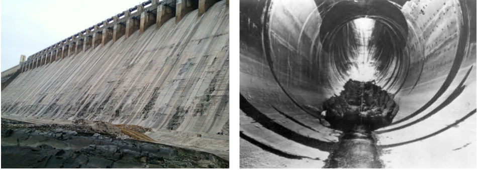
Figure 1.5: Effects of cavitation on hydraulic structures. Left: Nagarjuna Sagar Dam, India [Giridhar et al., 2014]. Right: Hoover Dam, USA [Warnock, 1945].
