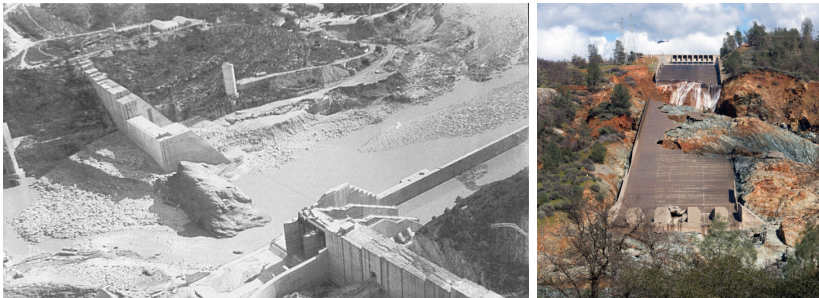
Figure 1.2: Left: rests of Tous Dam (València) after its failure in 1982. Right: state of the Oroville Dam (California) after the 2017 crisis.
