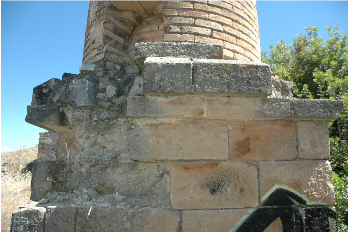
Fig. 4. Damaged stonework in the base of a chimney in Linares (Spain).
