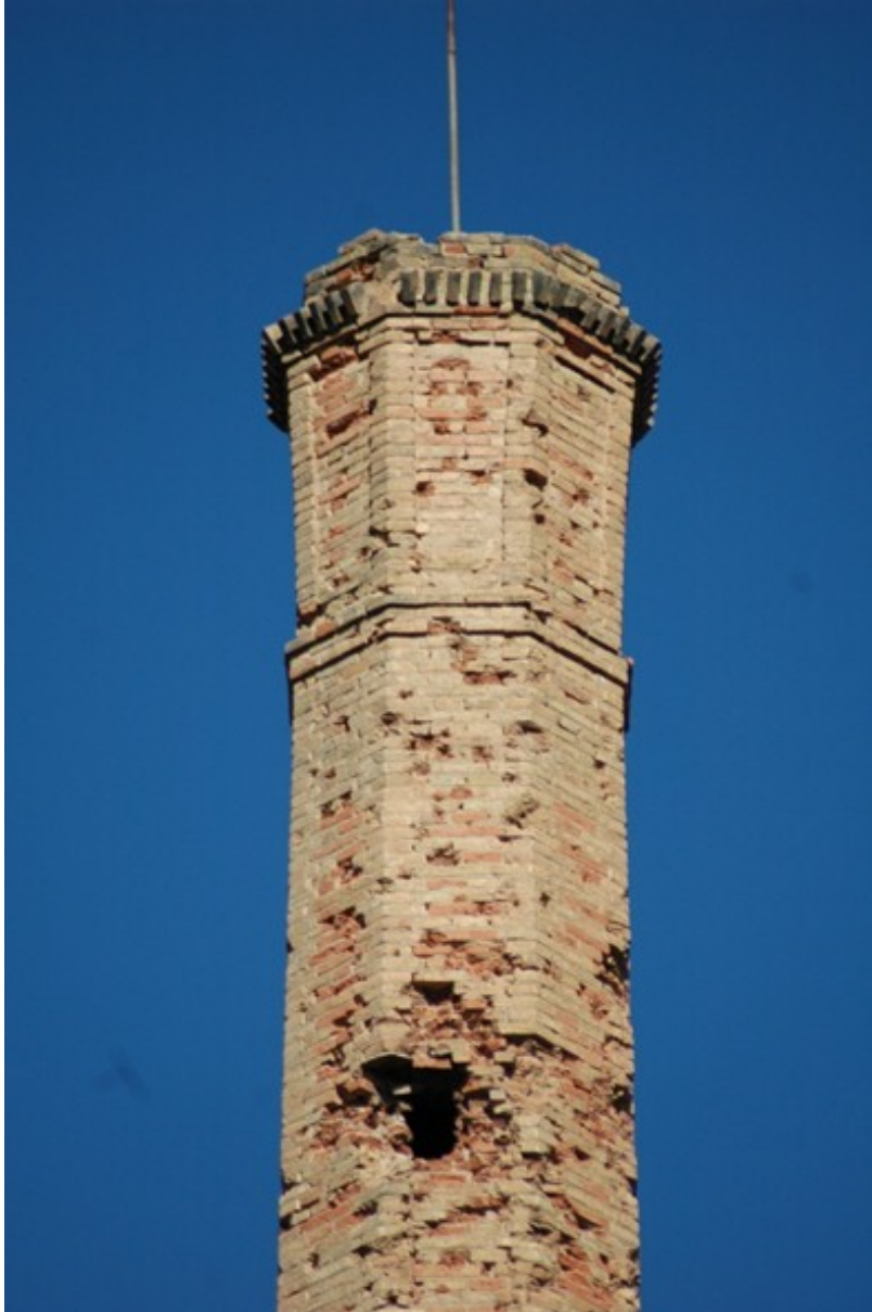
Fig. 14. Chimney in Teruel (Spain) damaged by artillery shells.
