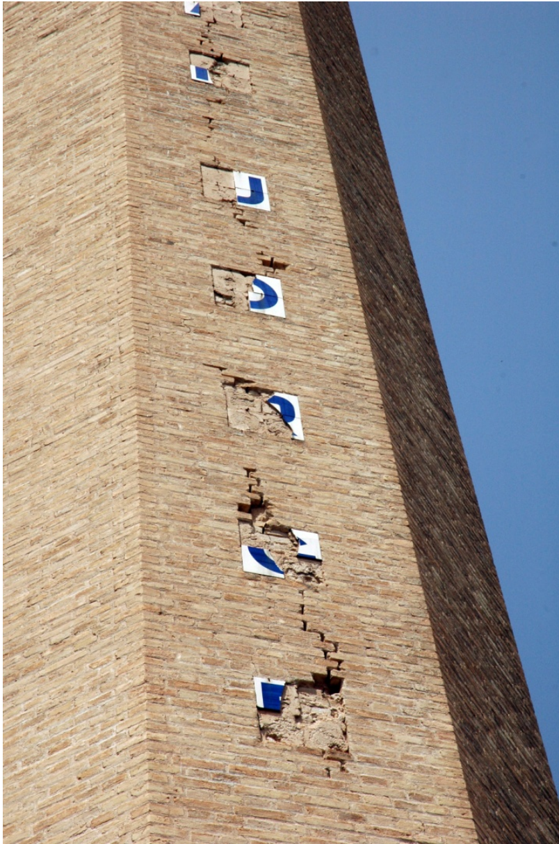
Fig. 6. Damaged decorative tiles in a chimney in Xàtiva (Spain).
