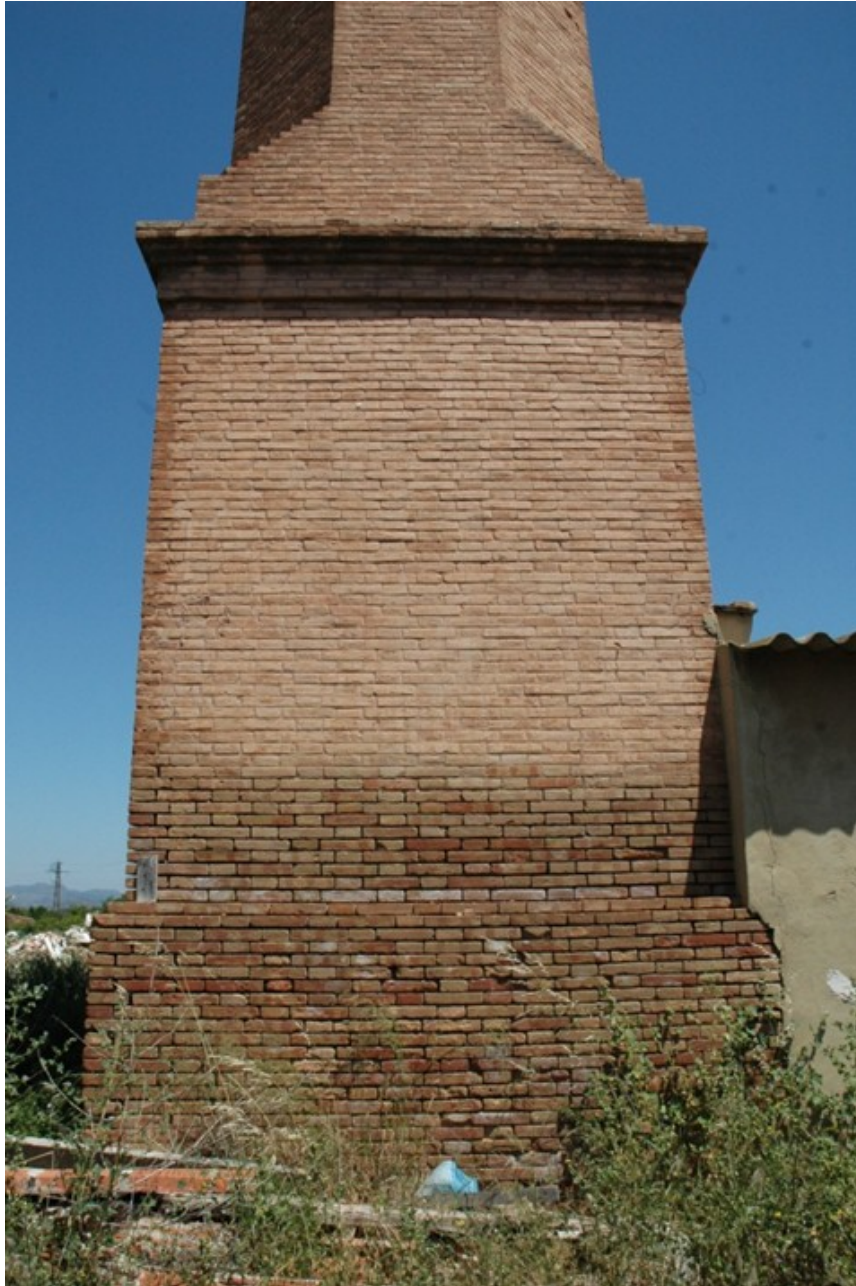
Fig. 11. Damp stains on the base of a chimney in Alfara del Patriarca (Spain).
