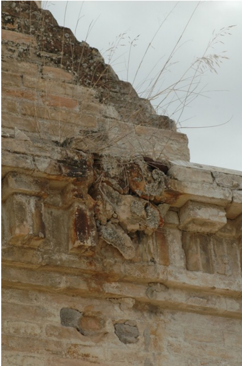
Fig. 17. Damage caused by growth of plants in the base of a chimney in Gandía (Spain).
