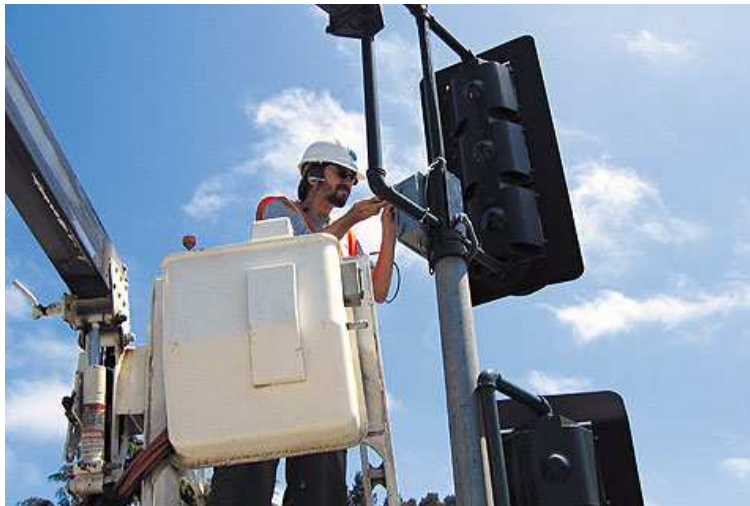
Figure 3.7: Example of an RSU installation.
