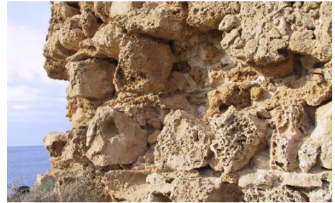
Fig. 4 - Inland side of the tower: evidences of tafones and flakings
