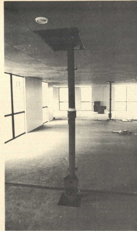
3 The essential flexibility I: the contractor moves out leaving a single volume with independent services (Montereau, France).
