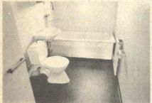
18. Typical Swedish bathroom. Note disintegrated appliances and gap between bath and wall. Bath drains into floor gulley. Single swivel h & c between bath and basin.
