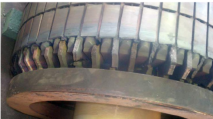
Fig 1. Rotor of a 5 MW, 6kV cage motor with multiple broken bars.
