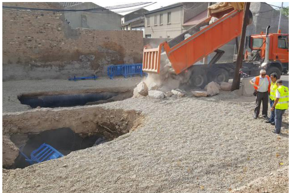
Figure 2. View of collapsing sinkholes that appeared next to C. de la Estación Street in August 2016.
