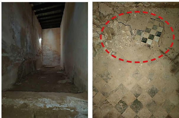
Fig. 25. Effect of moisture on the walls and deterioration of mosaic pieces in the vestibule. (Source: The authors).
