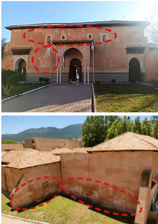
Fig. 24. Signs of disintegration and flaking of plaster and coatings on the exterior façades of the building. (Source: The authors).
