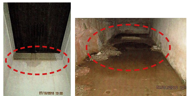
Fig. 23. Rainwater leakage through the roof and the formation of water puddles (photographs taken in 2016). (Source: Interpretation Center with a Museum-Oriented Character Dedicated to Algerian Costume and Traditions, 2018-2019).
