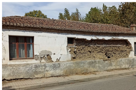
Fig. 8 – Kavaje: building after the 2019 earthquake, the collapse of the plaster shows the layer of earthen bricks and the thick layer of cement plaster; the roof does not excessively overhang (Rescic, 2023).
