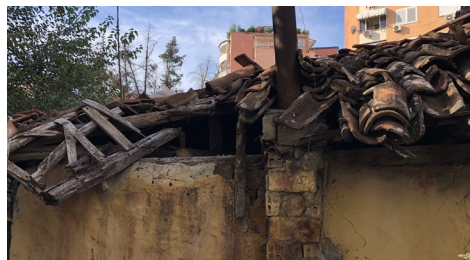
Fig. 10 – Tirana: building where roof is torn off (Luvidi, 2024).
