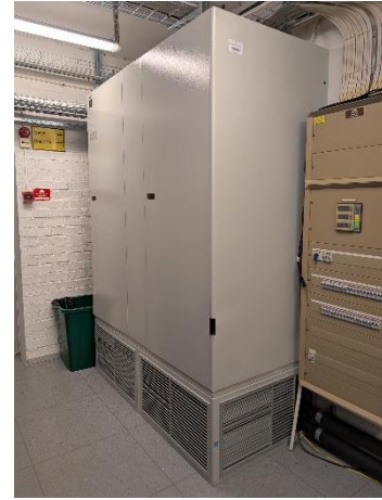
Figure 13 CRAC unit at PDC.
