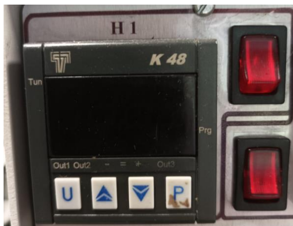
Figure 13. Furnace control panel.
