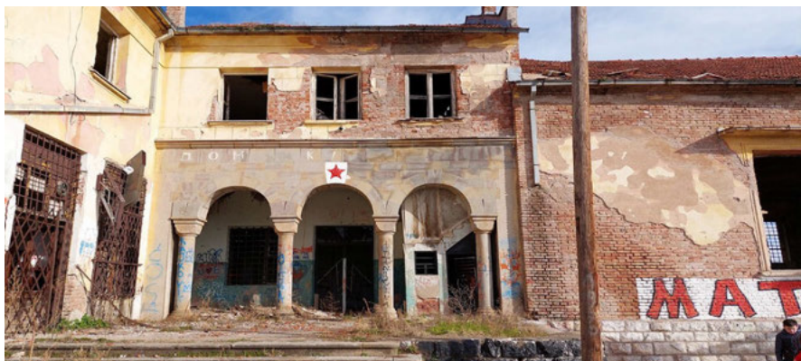
Figure 1. An example of an abandoned cultural centre in a village in southern Serbia. Source: (Author 2023)
