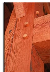
Fig.15 Joint photograph [Appalachian+woods, 2025]
