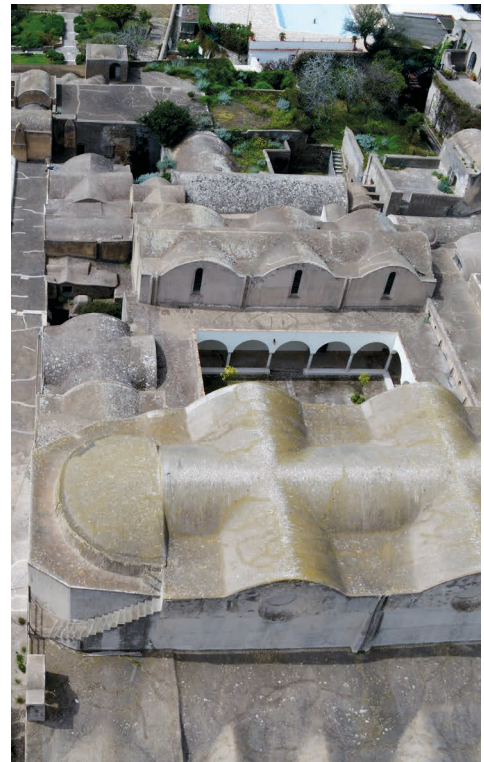
Fig. 3 – Extrados vaults of Chartreuse of San Giacomo in Capri. It's evident the presence of different forms of degradation on roof surfaces and, at the same time, the different kind of cementitious integrations (Facchini, 2018).
