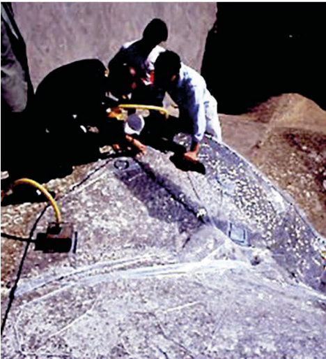
Fig. 2a & 2b – Two slides of 1980's intervention on extrados vaults system (Photographic Archive of Suprintendence of Naples, slides 017A, 067B).
