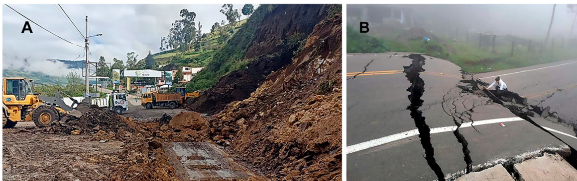
Figure 8. (A) Government machinery works to clean and clear debris to open the E-35 Road, South of the Don Fausto restaurant, in the Casual sector, 19 February 2023 [30]. (B) Impressive open cracks and vertical displacement (over four meters) 50 m North of the Don Fausto restaurant. The picture was granted by S. Berrones, a geologist, who took it on 26 March 2023, in the morning, a few hours before the event happened.
