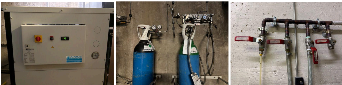
Figure 37. (From Left to right) Water, gas and compressed air streams for the HP furnace
