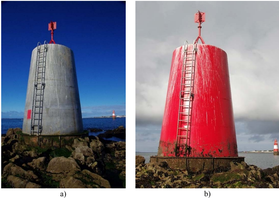
Figure 6. a) turret condition in September 2013, b) condition in September 2015 after final paint application and two winters. Pictures E. Denarié.
