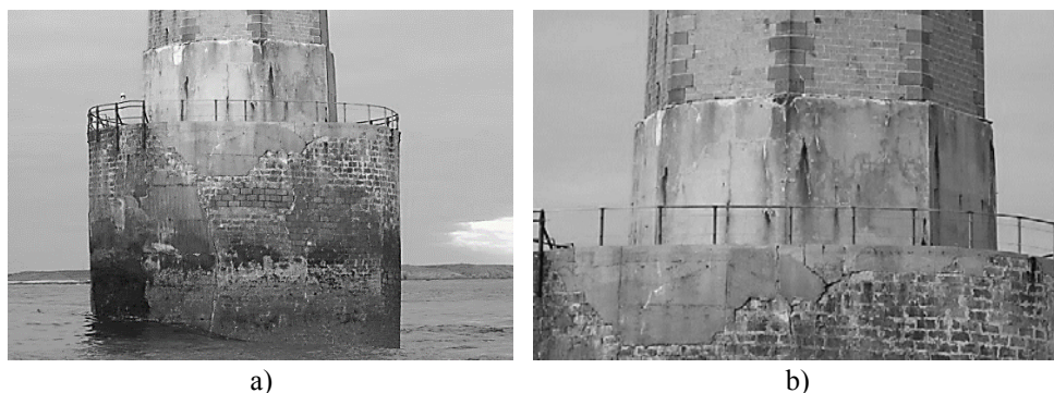
Figure 3. “La Jument” lighthouse, Ushant, France, condition in 2013: a) basement, b) Reinforced concrete reinforcement ring at the base of the tower, made in 1918, photos E. Denarié.
