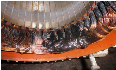
Fig. 7. Insulation damage occurred in 2010 in the same motor due to catastrophic failure of the bearings.
