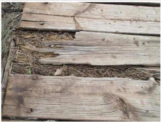
BROKEN WOODEN PLANKS IN THE PATH ADAPTED FOR DISABLED PEOPLE
