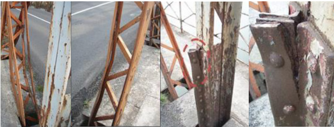
Figure 5. Deformations and breaks due to impacts
