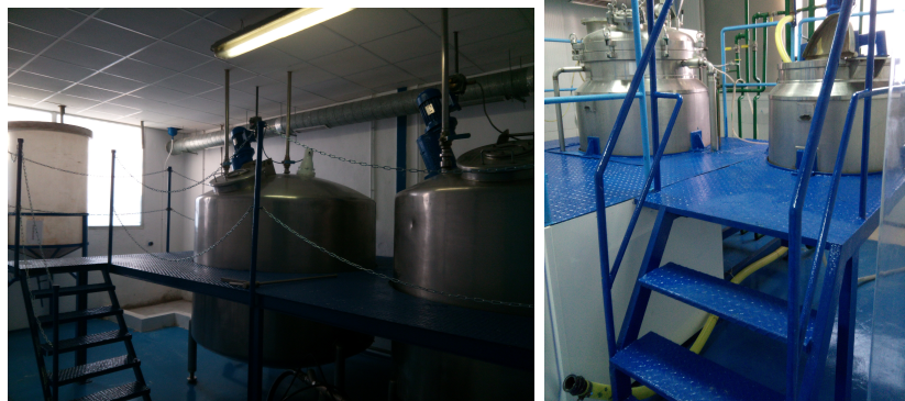
((c)) Sala reactores
