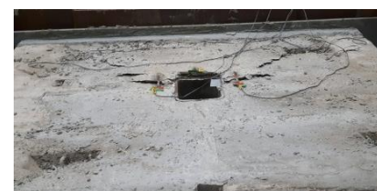
Fig. 12. Shear cracking of slab of specimen SP6
