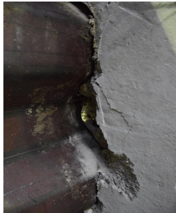
Fig. 9. Concrete crumbling at the web-to-slab connection (P17-T-14).
