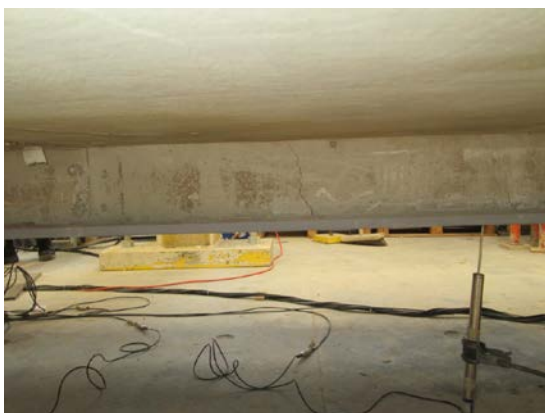
Fig. 9. Shear cracks in SBT1a from previous test series.
