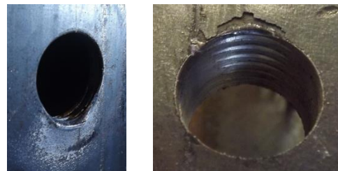
Fig. 11. Observed damages (P3.1-1)
