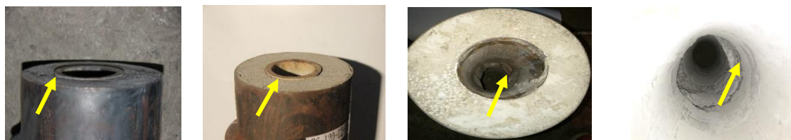
(a) Bamboo sprung back. (b) Buckling of inner steel tube. (c) Crushed concrete.
