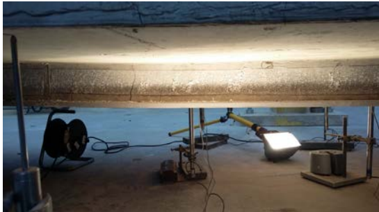
Fig. 7. Concrete cracks around beam web for BT7
