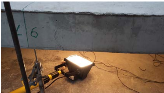
Fig. 8. Concrete cracks on outside edge of lab for BT7
