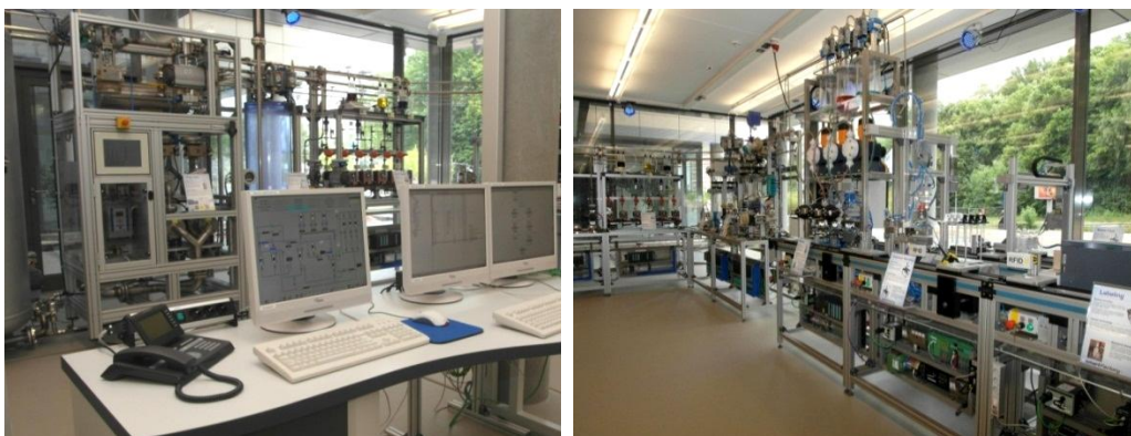
Figure 13: View on the demonstration plant SmartFactory KL
