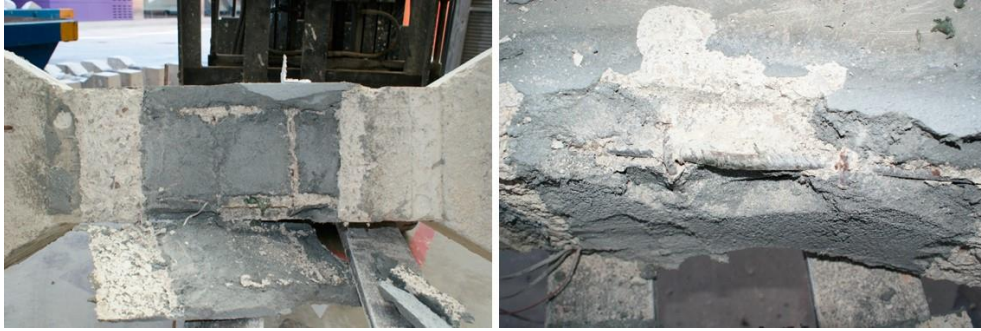
Fig. 11. Column failure: Specimen P4W (repaired column with R4-mortar and no BA). Detail of the detachment of the patch
