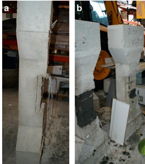
Fig. 4. a) Detail of the column hollow to perform the patching repair; b) Filling the first layer of column patching
