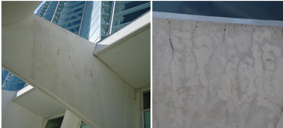
Fig.15. Cracks in cantilever beams
