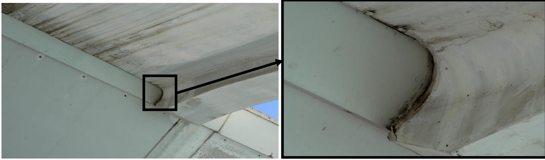
Fig. 3. Damp in stairs-slab joint (left) with detail of most affected zone (right)
