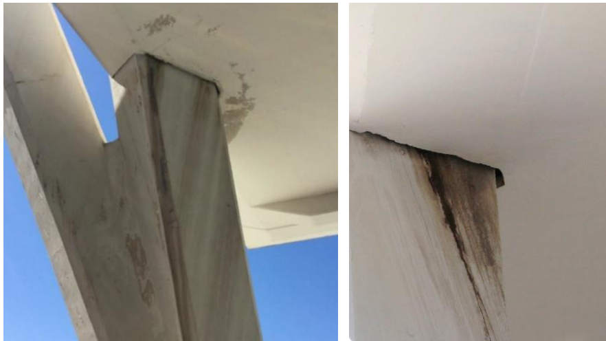
Fig. 1. Damp patches in column-slab joints
