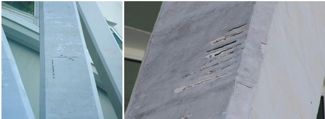
Fig. 12. Corrosion of column reinforcement
