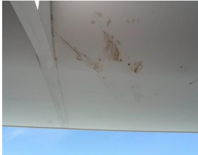
Fig.9. Rust stains due to water leaking through a floor slab
