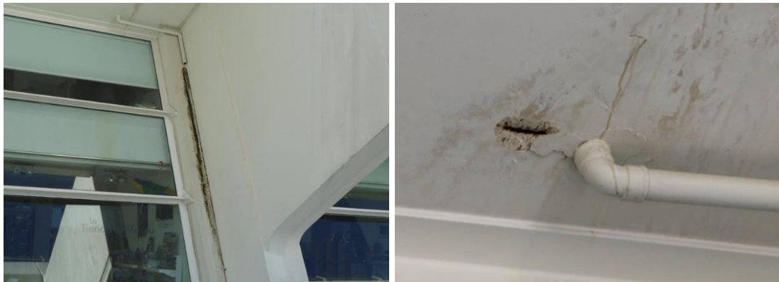
Fig.8. Deficient rain drainage on exterior wall. Generation of aesthetic defects (left) and corrosion of reinforcement (right)
