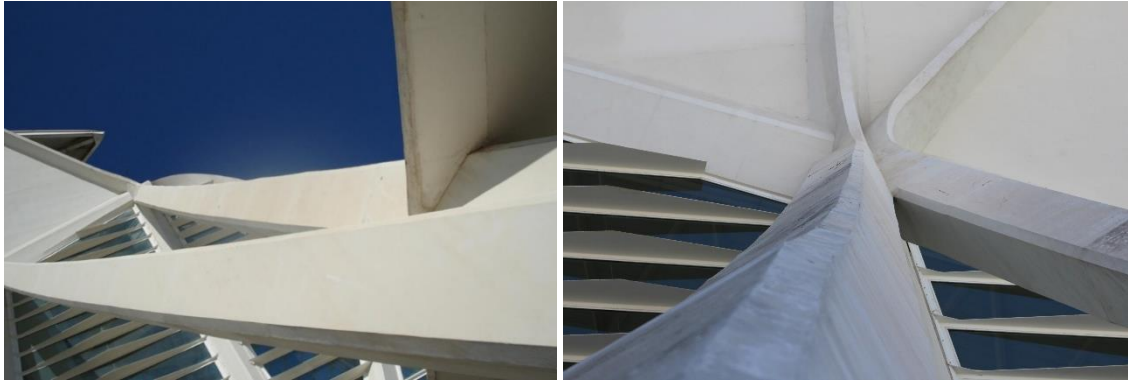
Fig.19. Deformation of columns at front and rear of the building.
