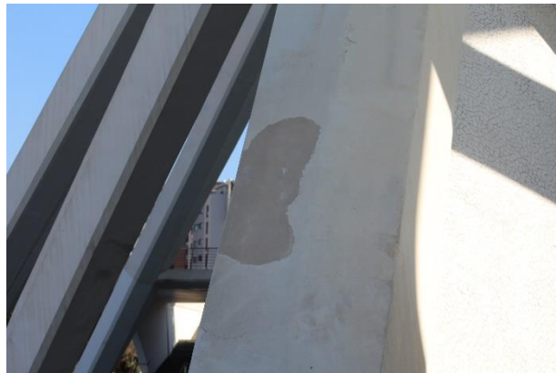
Fig. 22. Mortar patches on columns
