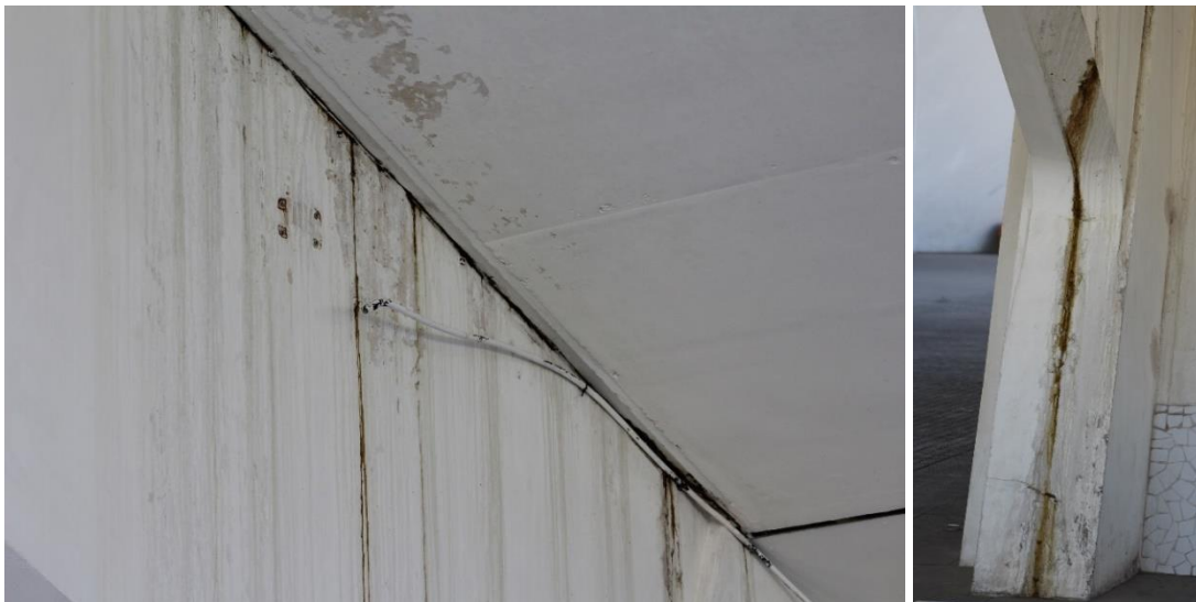
Fig. 2. Damp in wall-slab joint (left) and on base of wall (right)
