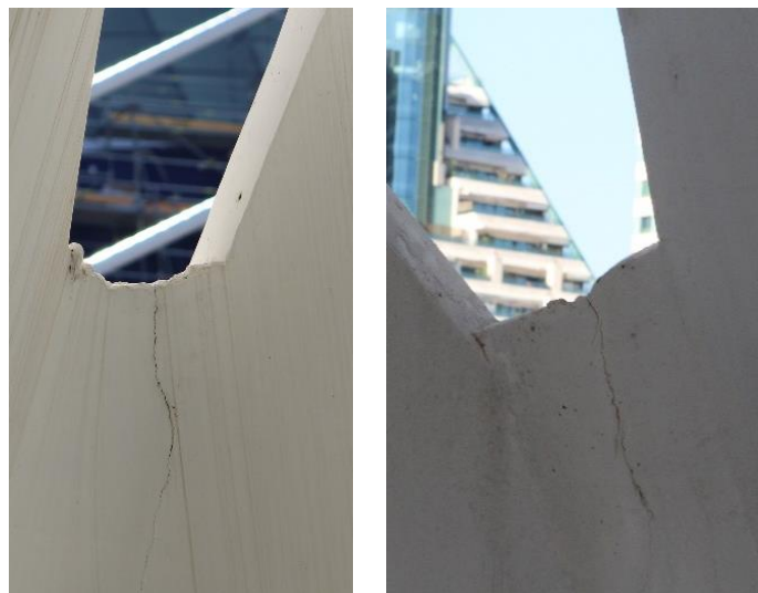
Fig.18. Cracks at the point where two columns meet
