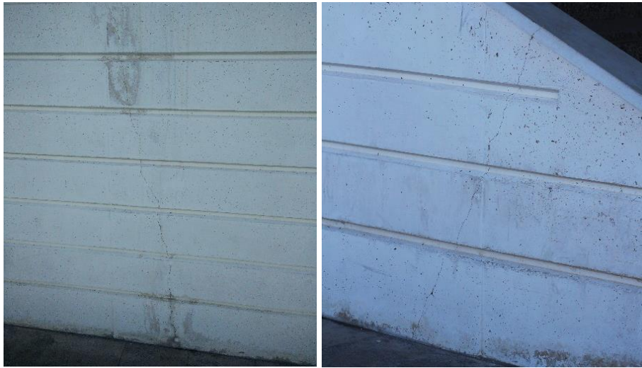
Fig.13. Early age thermal cracking in a wall
