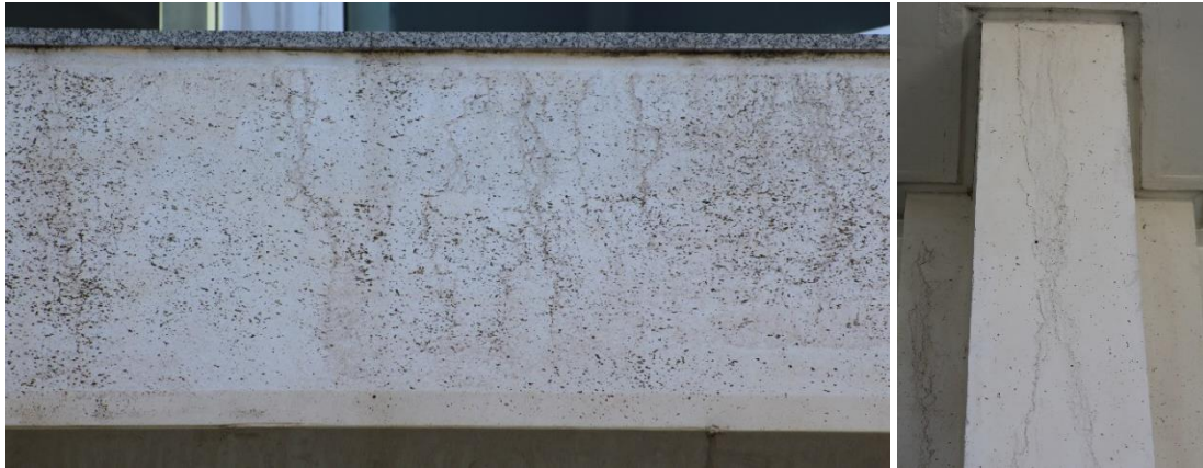
Fig.11. Surface pores in cornices (left) and columns (right)
