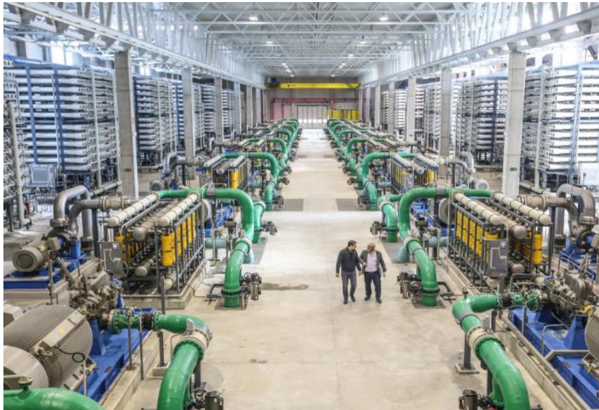
Figure 20. Torrevieja Reverse Osmosis phase where can be observed the big RO trains connected to the high pressure pumps and the pressure exchangers ERDs. [38]
