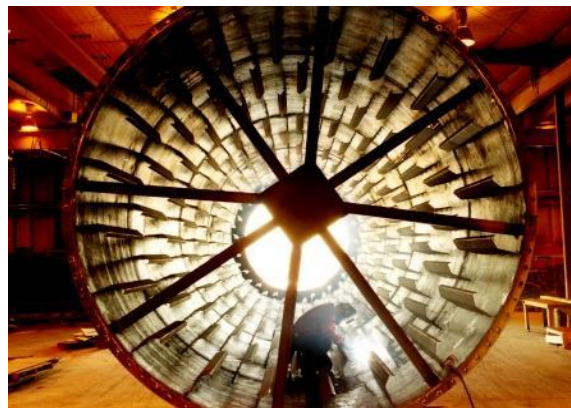
Figure 21 Rotary Dryer Drum
