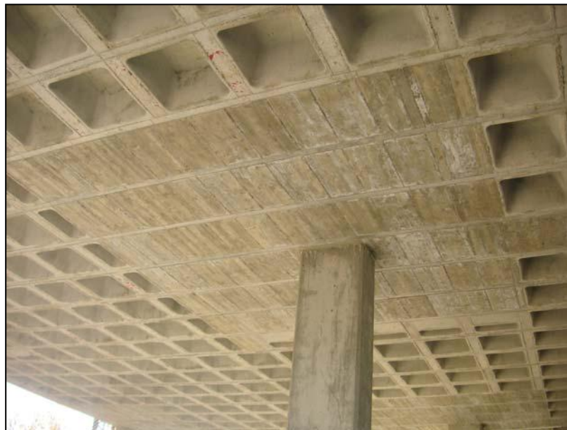
Picture 4.3.2.1: Bottom waffle slab where the caissons are observed and the abacus on the pillar. Source: http://www.celsa.com
