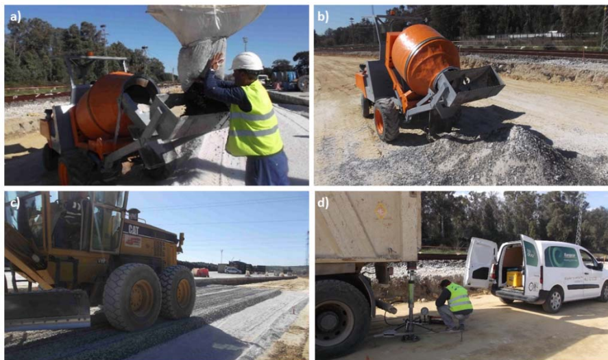
Figure 4. Construction process. (a) Mixing process of the rubber-aggregate mixtures. (b) Subballast placement after mixing. (c) Subballast extended using a motor grader. (d) Static load plate test.
