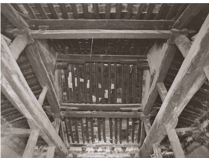
Fig. 40| Interior construcción, método tailiang Fuente: Zwerger, K., Olgiate, V. (2012) Wood and Wood Joints : Building Traditions of Europe, Japan and China
