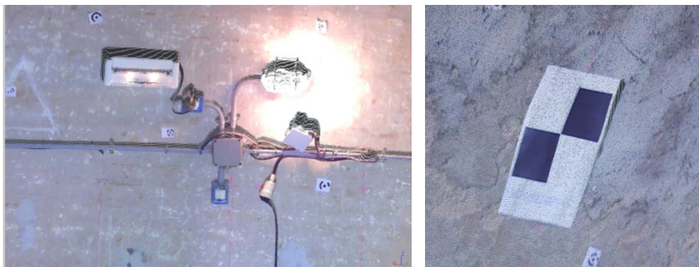
Figure 7.39. Example of the electrical installation and targets to be deleted (3DReshaper)
