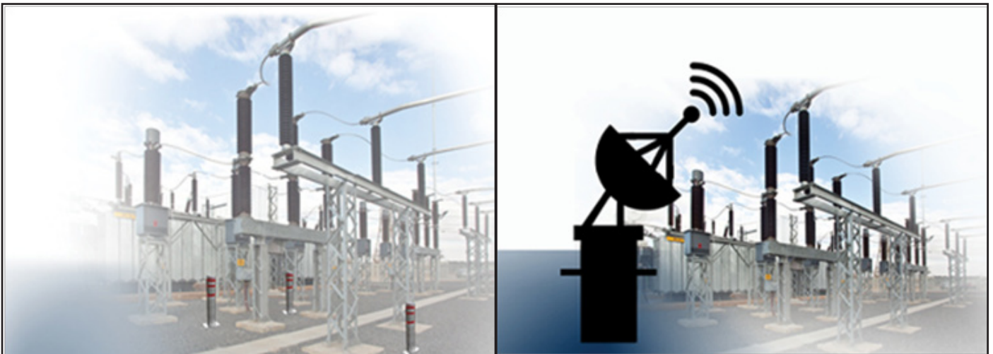
Figure 18. Sensors placed in each hotspot Figure 19. Radar in the middle of the substation
