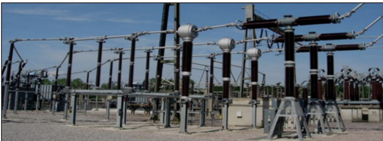
Figure 1. View of an electric substation
