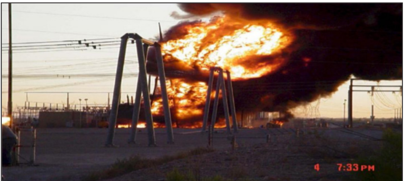
Figure 2. Explosion of a transformer in a substation
