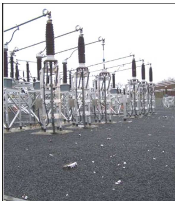
Figure 3. Scattered parts after an insulator explosion
