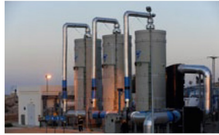
Figure 41 – (12) Odor control (SUEZ, 2017)
