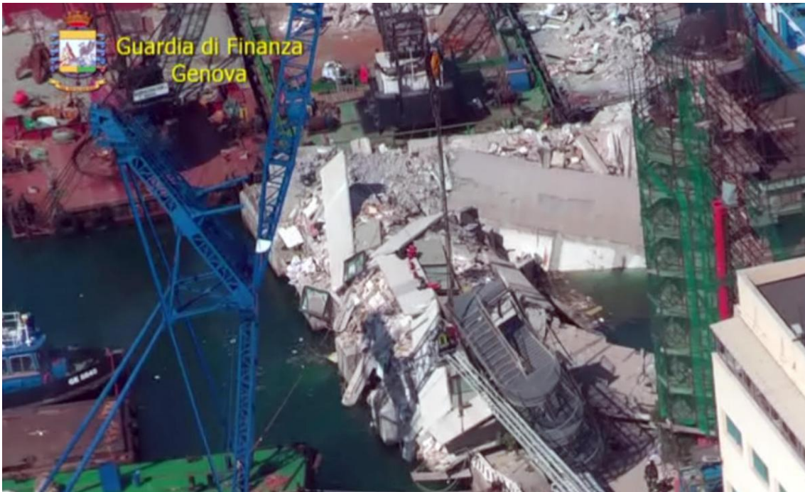
Figure 1-5 Effects of the impact of the cargo ship “Jolly Nero” against the mole of the Genova’s dock.
