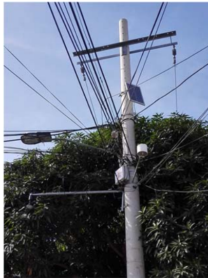
Figure 9. Monitoring, Communication and Power supply system of an EWS for urban flash floods in Barranquilla (Colombia)
