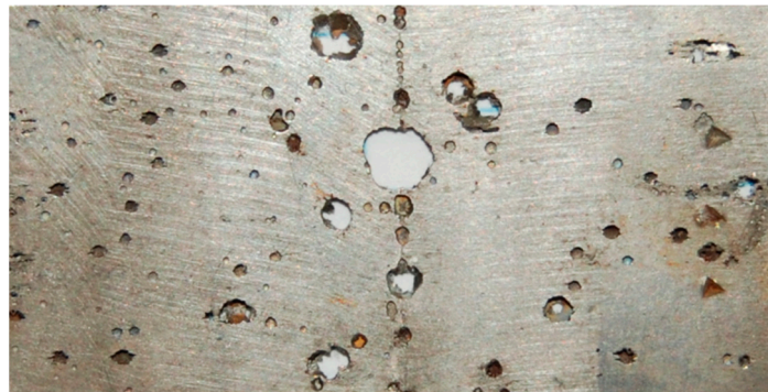
Figure 10. Pitting at the welding and HAZ zones of a 33% cold work sample.
