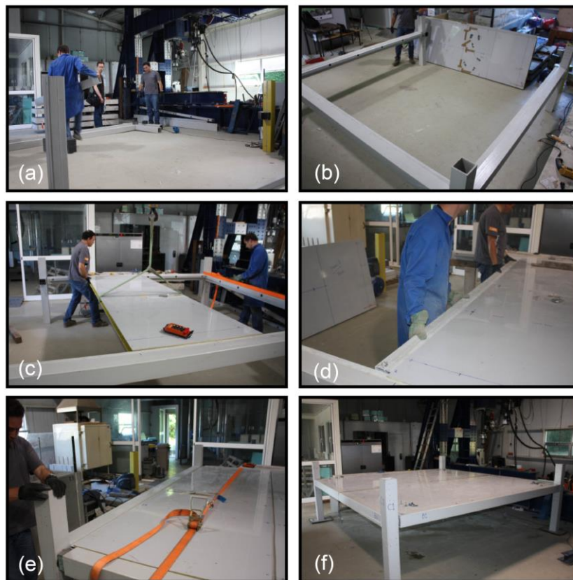
Fig. 3. Stages of the assembling process: (a) placing columns; (b) connecting beams to the columns; (c) mounting panels along beam-panel connection; (d) placing panel-panel connector; (e) installing the last beam; (f) final prototype.
