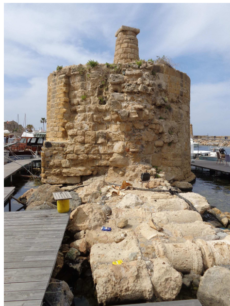
Fig. 1. Roman stone column bases were recycled for the foundations of the dock (Photo A. Camiz, 2018).
