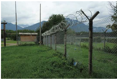
Fig. 3. Part of the damaged fence of Site Rigel, Naz-Sciavez. (Author, August 2019).
