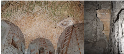
Fig. 15. Panoramic view of the cross vault with an opening for access to the roof-level and the preserved stone corbel (authors, 2019).
