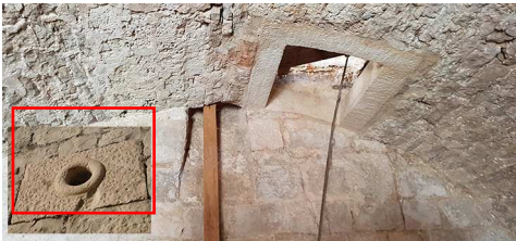
Fig. 11. The ground floor vault with the opening from the upper floor and ventilation channel with its outside outlet (authors, 2019).
