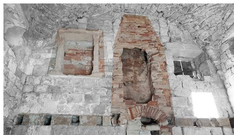
Fig. 13. Visible holes for the beams' support structure between the first and second floor, stone sink and fireplace (authors, 2019).
