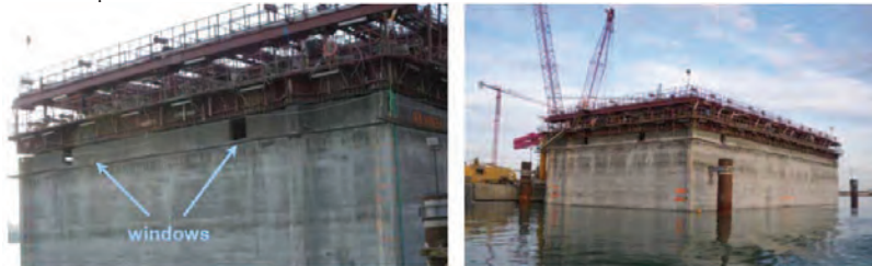
Figure 8.- CYES floating dock facility
