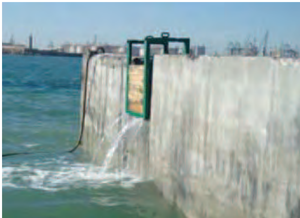
Figure 10.- Cap used for closing external windows in caisson.
