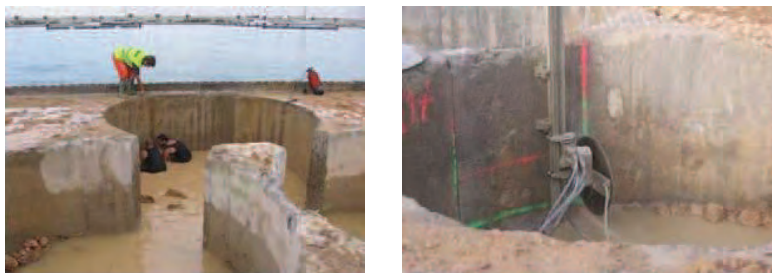
Figure 1.- Construction of wave-dissipating chambers, (a) circular cells and (b) diamond wire cut.
